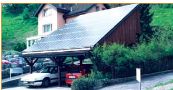
Roof-mounted System 6.0 kWp
