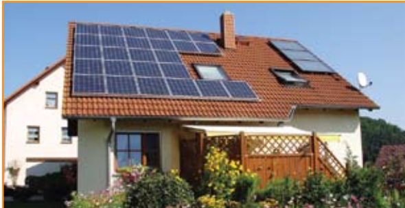
Roof-mounted System 5.1 kWp
